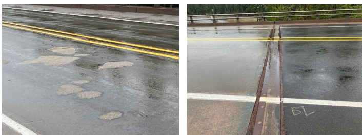
Current conditions of the damaged bridge deck surface on the OR 35 overpass at U.S. 26.
